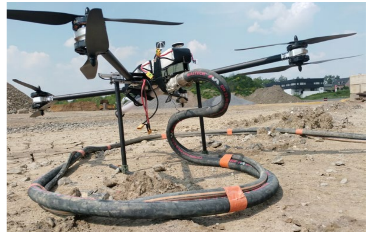
Fig. 10. Thick mortar sprayer pipe connected to the drone for constant material feed.
